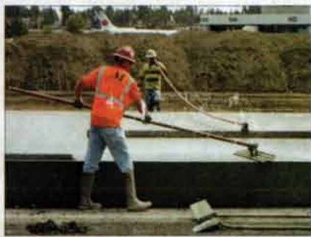
Workers smooth a recently poured 18-inch deep section of runway Tuesday at Sea-Tac Airport. The longest runway is being torn up and simultaneously replaced.
